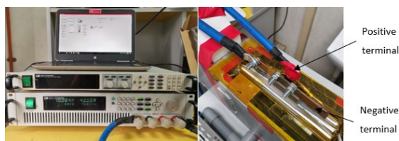
Figure 4: Battery connection to electronic load
